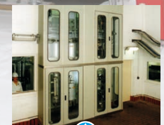
A special gas-tight shelter for a toxic gas plant.
