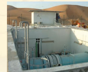
Extreme insulation and passive cooling allow this pump control and instrumentation shelter on a desalinated seawater pipeline network to operate by solar power alone. GRP with gelcoat surface provides durability for the harsh Middle East coastal location with chlorine, UV and dust/sand.
