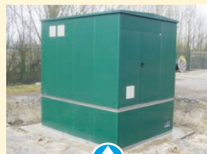
Equipment shelter above a gas cavern storage facility.
